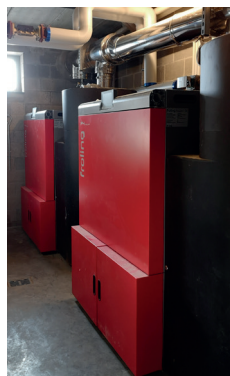
Chaufferie 2 X 100 kW
